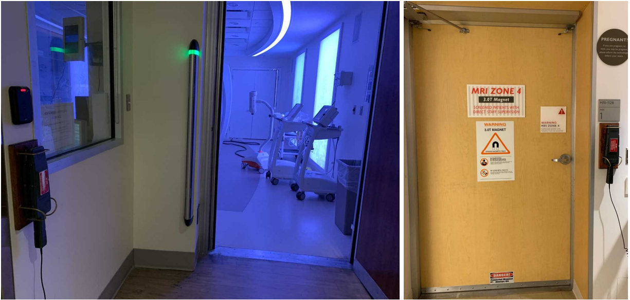
Figure 1: On the left a secure MR doorway with FMD and the 5G line demarcated by floor color change and roof lighting. On the right, an example of the secure PET/MR door with zone 4 signage, wall mounted FMD and pregnancy sign. Images courtesy of New York-Presbyterian Cornell Weill Medical Center and Memorial Sloan Kettering Cancer Center.
